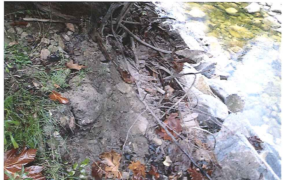
CK2235 Left Abutment fill slumping
